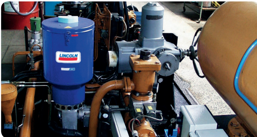
For hydro-electric power plants and turbines that are in service around the clock, a reliable lubricant supply is indispensable
